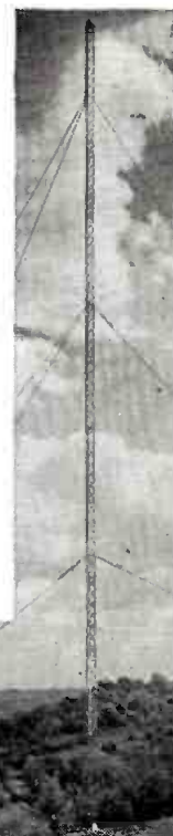
Slender 275-foot insulated tower for AM radio
